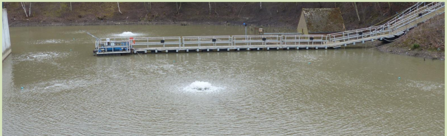
Below. Multiple diffusers used in conjunction with 1hp Splash surface aerators in a landfill site lagoon. System requirements were to strip harmful gases, and improve discharge water quality. Improvements were seen on day one, with a drastic reduction in ammonia levels.
